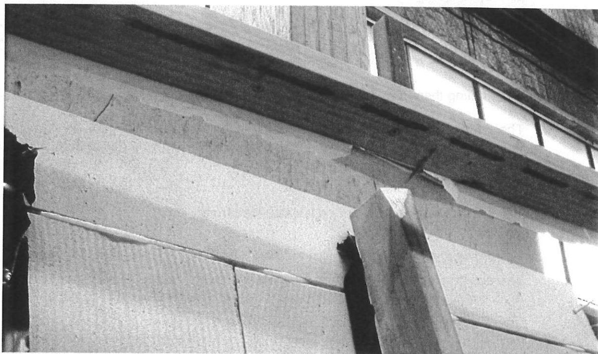
Figure 5. Separation of studs from the top plate
